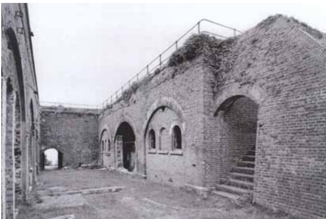
The Guard House range, and steps to the terre-plein, from the north-east, photo taken 1998 (NMR: BB99/15911)
