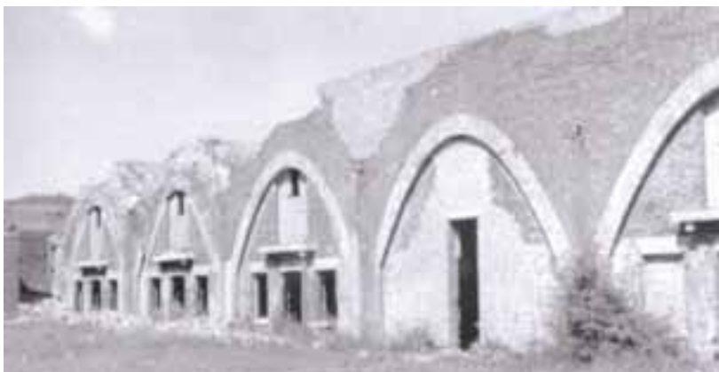
The Soldiers' Quarters at the Drop Redoubt, photo taken 1958/9 (d07905 Dover Museum)
