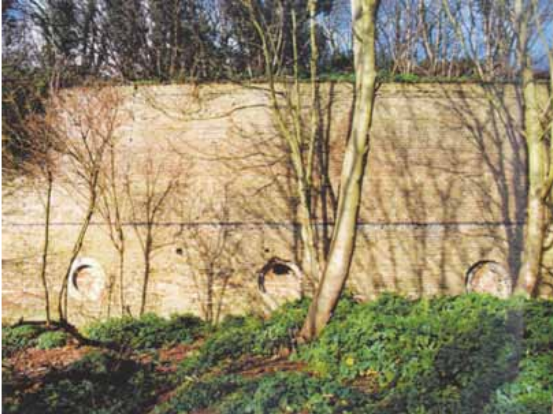
The infilled northern end of the South Entrance Ditch and the smoke vents of the casemates behind the northern scarp revetment, looking north, photo taken 1998 (NMR: AA00/8595)
