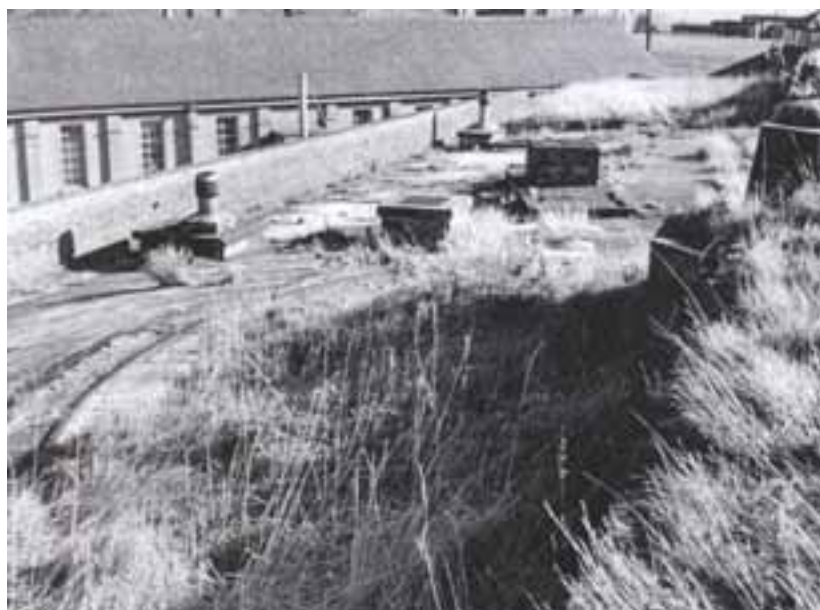
The terre-plein of the western face in the Citadel, showing a racer from a traversing gun platform and embrasures in the parapet, before their removal or concealment, photo taken 1959 (A5513/34 Dover Museum)
