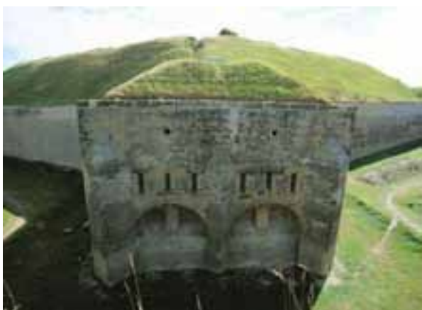
The Drop Redoubt's Caponier no. 3, showing the northern face wall, photo taken 2005
