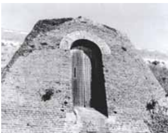
The reinforced two-leaf door which led onto a bridge to the tenaille, photo taken 1998 (NMR: BB032740)
