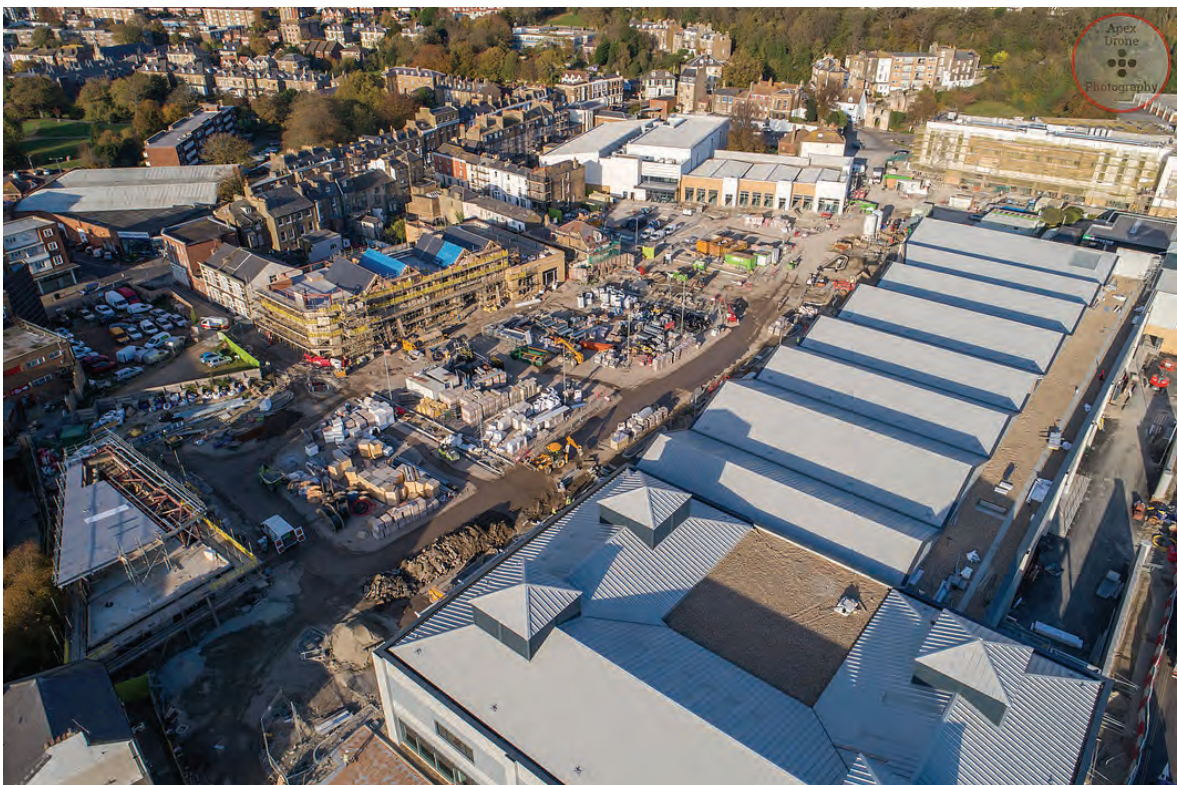
Figure 11.4 Aerial view of the St James's site in progress (Photo courtesy of Apex Drone Photography)
