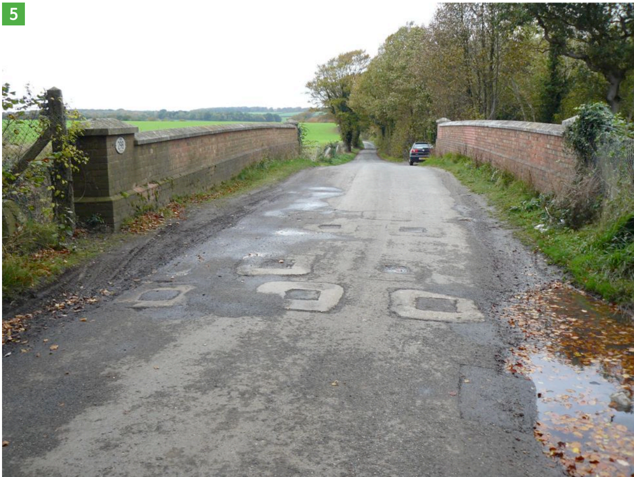
5. Scars in the road mark the position of a Second World War road-block on a bridge over the Dover to Canterbury railway line.
