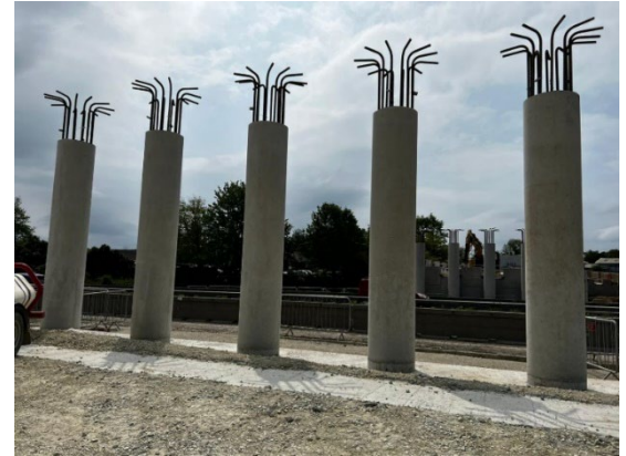
Image: Construction of concrete columns for the bridge in Section 1B North
