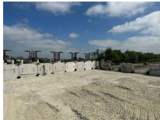
Image: Construction of walls for the bridge and embankment in Section 1B South
