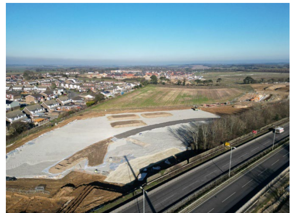
Construction of the trial embankments and temporary access road for the piling works - Section 1b North
