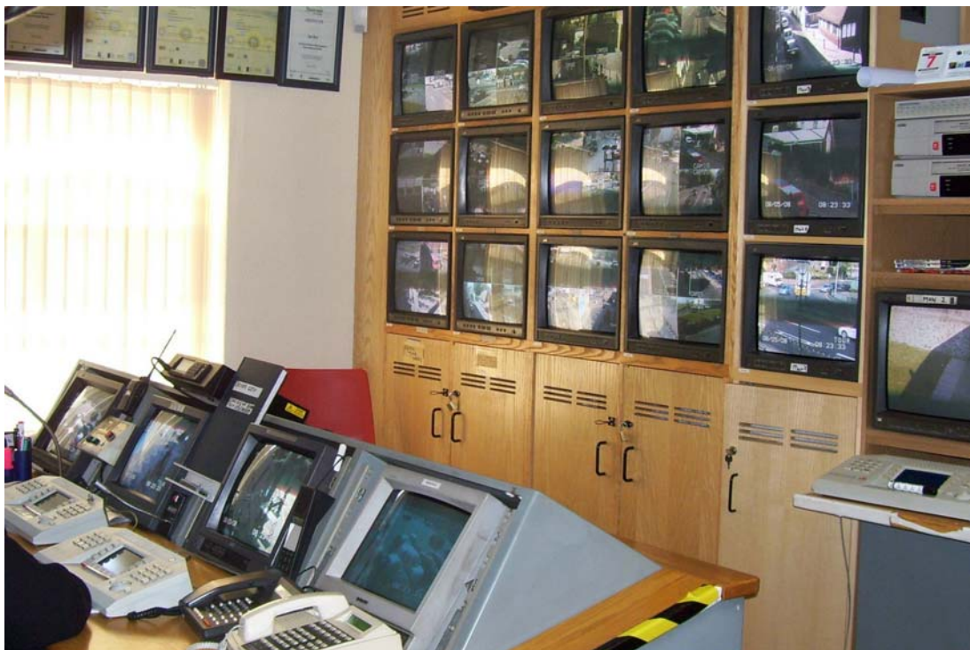
Dover CCTV Control Room
