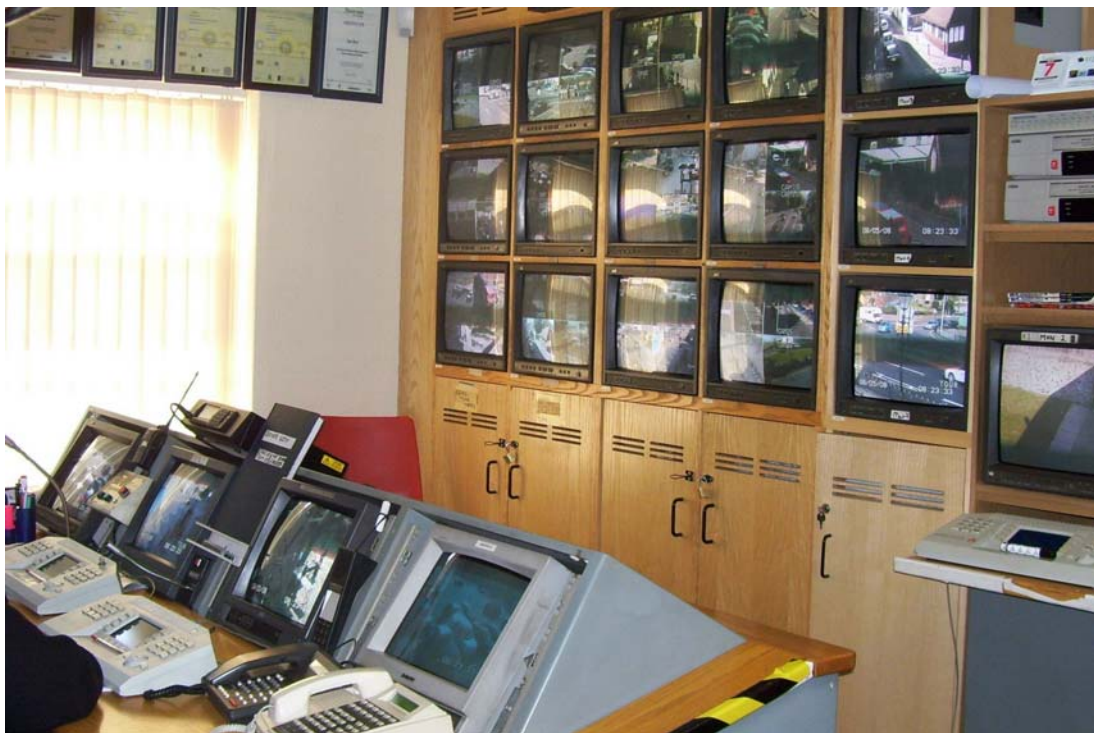
Dover CCTV Control Room
