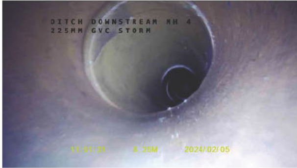
5, 00:02:19, 8.30 m Crack, circumferential at joint from 9 o'clock to 1 o'clock
