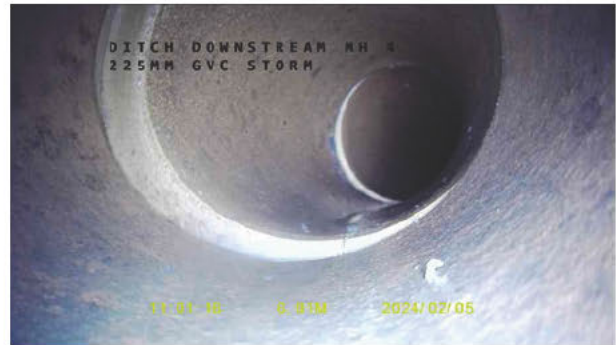
4, 00:02:03, 7.00 m Line deviates right, 15 degrees
