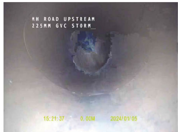
4, 00:00:28, 8.00 m Crack, circumferential from 12 o'clock to 12 o'clock
