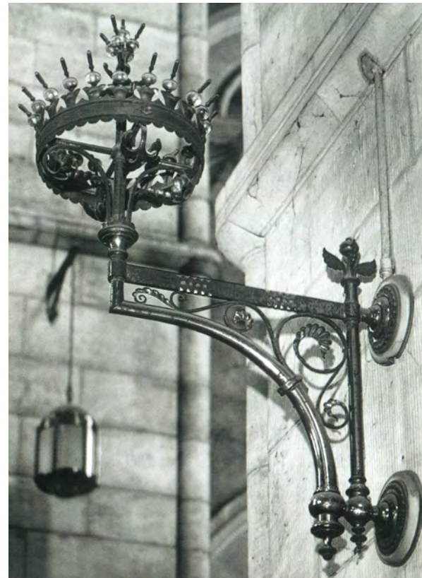
(c) Base plate to the gas brackets at Fin Barre Cathedral. (Internal ref: J Mordaunt Crook_174) [See App.01_Fig.3.10 for similarity of wall pattress plate]
