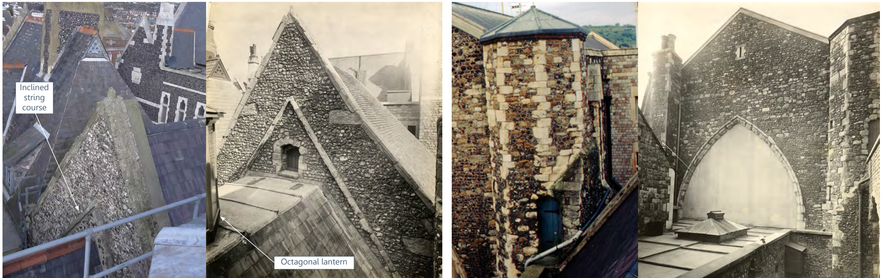
(a) Inclined string course on east gable of chapel. Current (Int ref: DSC05581) & historic (DMA ref: D30531)
