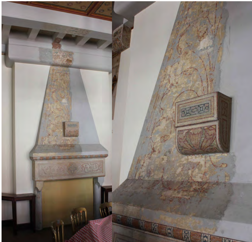
(a) Fire place in the Mayors Parlour at Maison Dieu (decoration partly uncovered) (Internal ref: IMG_5966 & IMG_5963)
