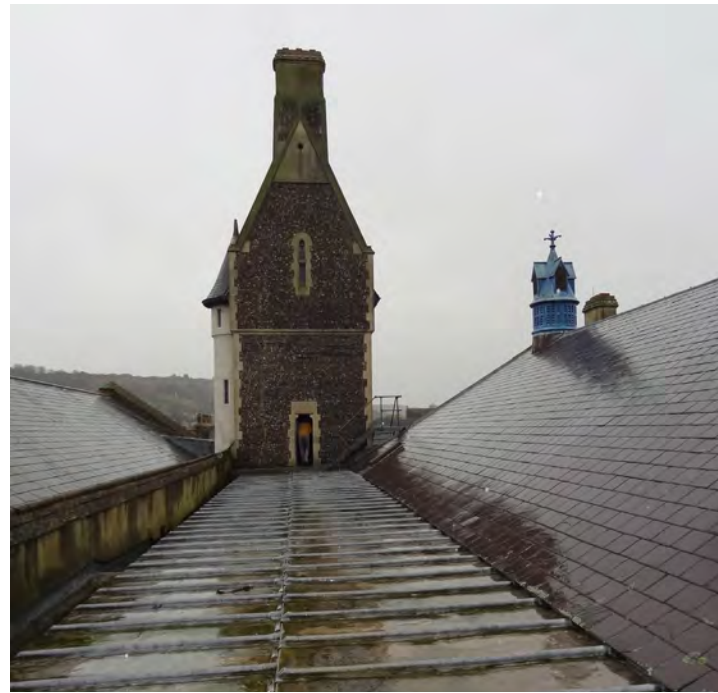
(c) Flat lead roof above Connaught Hall south gallery. Clock tower in distance and sun burner vent to the right. (Internal ref: DSC05011)
