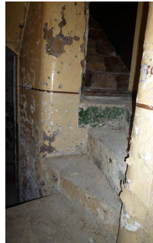
(g) Mediaeval stair turret treads repaired with Roman cement. View towards Tower GF (Internal ref: P1110081)
