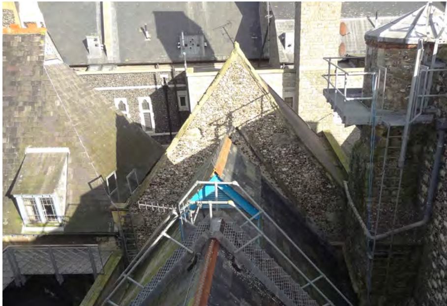
(d) Two roof levels over Sessions House. Note cupola on lower roof. (Internal ref: DSC05578)
