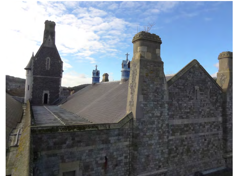
(c) Connaught Hall east gable and south roof slope with rear of Clock Tower in the distance. Stone Hall roof to the left (Internal ref: DSC05579)
