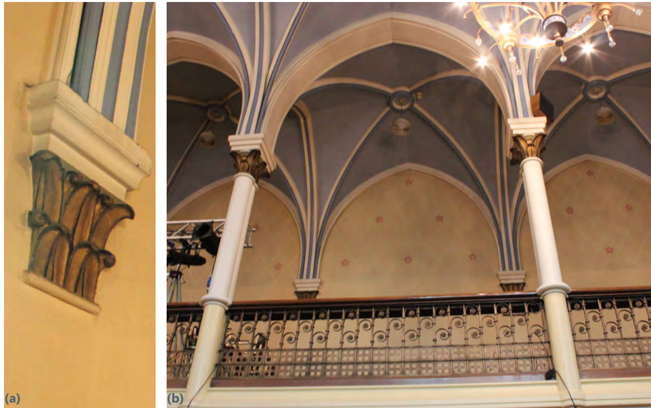
(a & b) Wall pilaster detail and Gallery space to the Connaught Hall. The star decoration is 20th century wall paper; Refer to Plate 25(a) for original decoration. (Internal ref: IMG_7596, IMG_7585)
