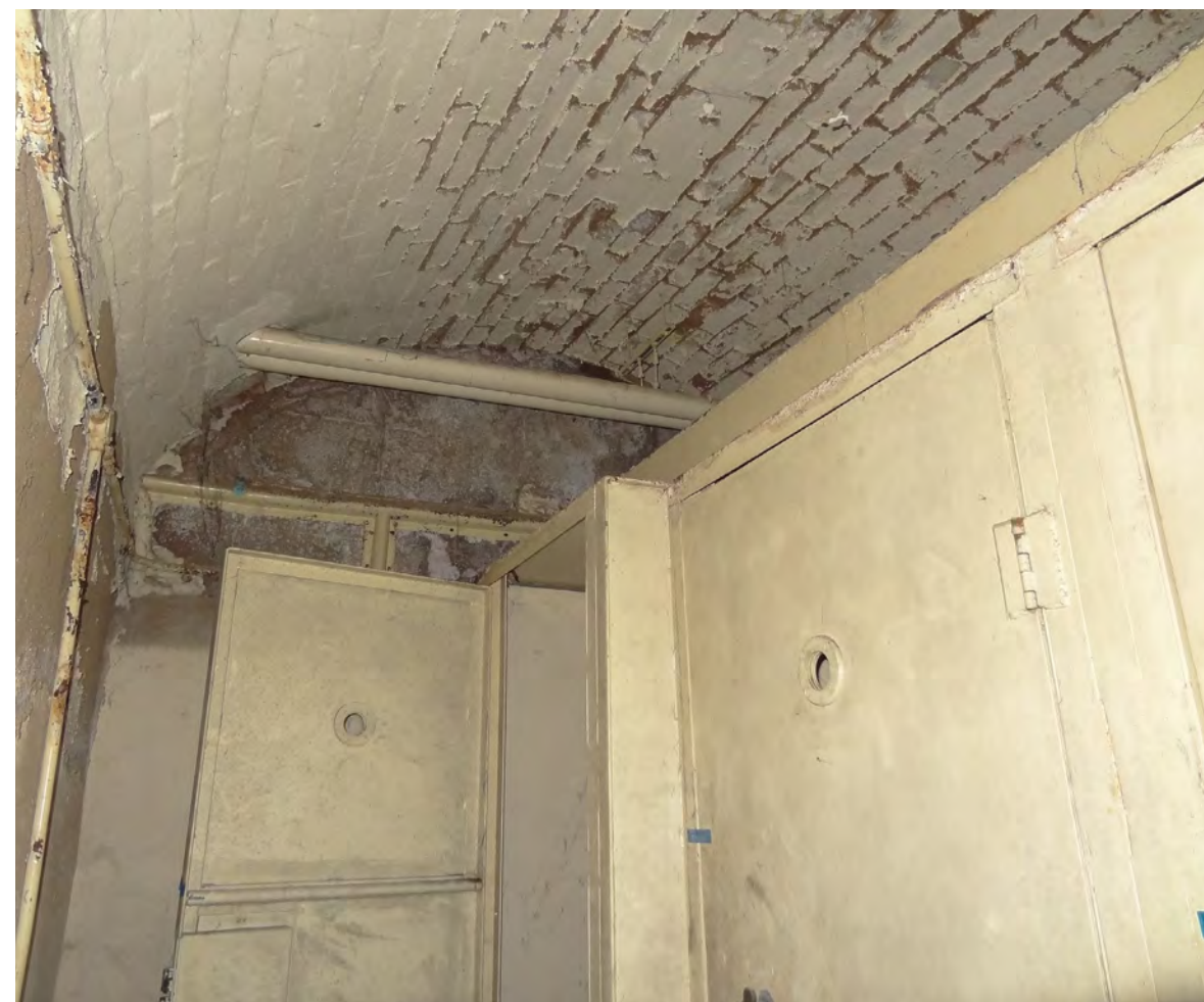
(d) Vault beneath Sessions House in east passage with early Portland cement render to wall. Note metal lock up cells with peep holes. (Internal ref: DSC05553)
