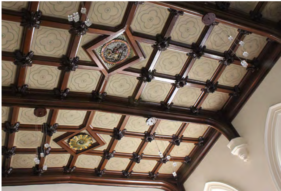
(a) Coffered ceiling to Sessions House within the original Chapel. (Internal ref: IMG_7091)
