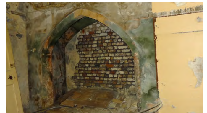
(k) unexplained arched recess between Museum Store and existing Chapel. (Internal ref: DSC05051)
