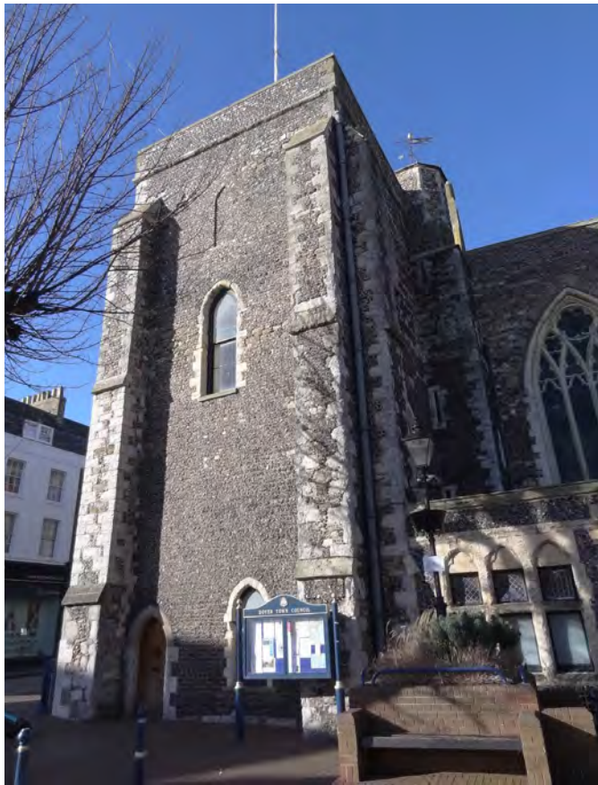
(a) South face of Tower. Note blocked upper stage opening. (Internal ref: DSC05654)
