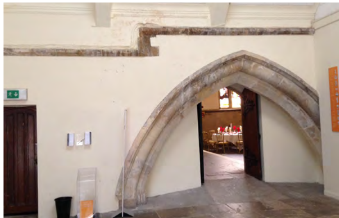
(e) South wall of Sessions House showing mediaeval arch and stepped string course. (Internal ref: IMG_0031)
