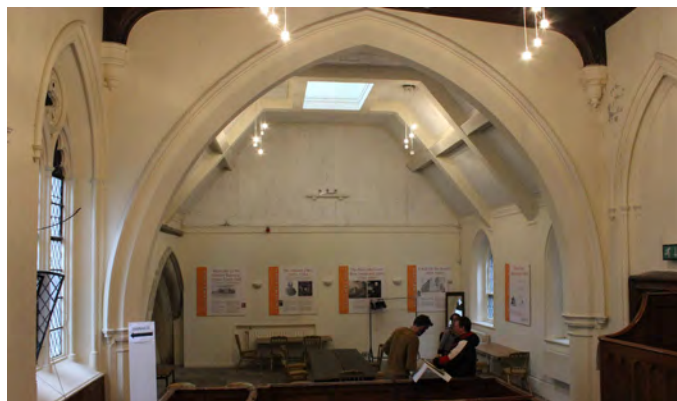
(f) Internal view looking west. Note roof lantern to lower roof. (Internal ref: IMG_8004)
