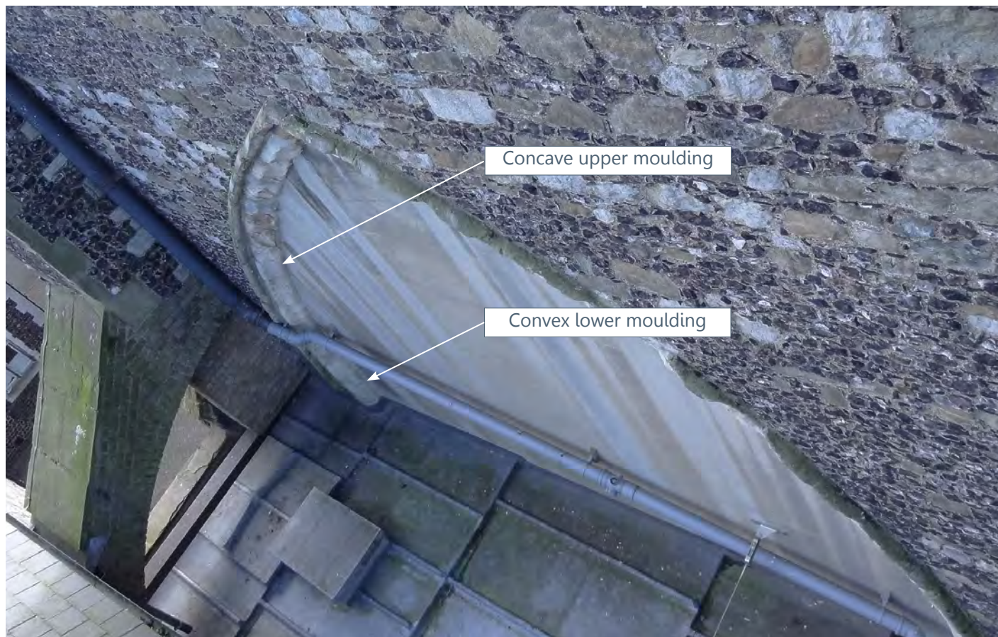
(d) East window moulding making a transition from convex moulding in jambs to concave in the arch (Internal ref: DSC05583)
