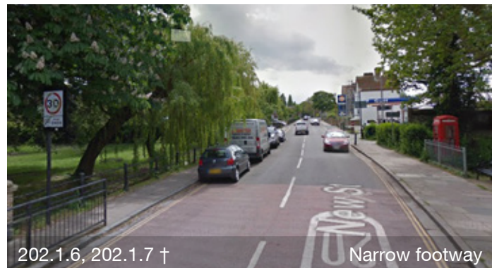
202.1.5 † Lack of continuous level footway
