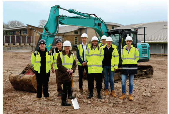
Figure 1 - Ground breaking 10 March 2026, with Cllr Lynne Wright, representatives from Alliance Leisure and Pellikaan
