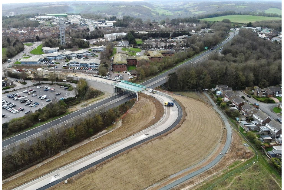
Image above shows Section 1b North (new bridge and embankment) and construction of asphalt.
