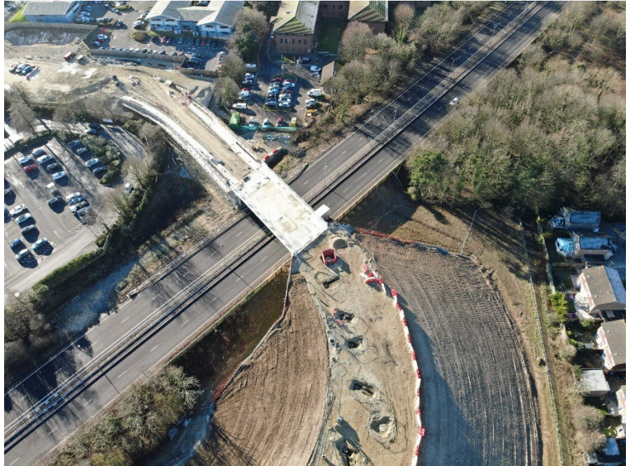
Image above shows Section 1b North (new bridge and embankment) and construction of gullies.
