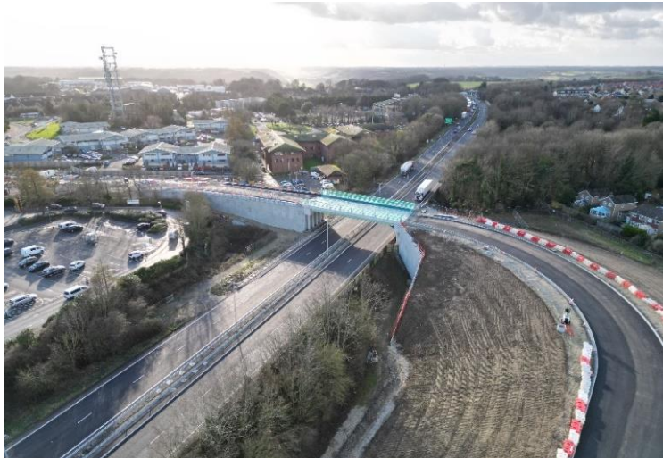
Image above shows Section 1b North (new bridge and embankment) and construction of asphalt.
